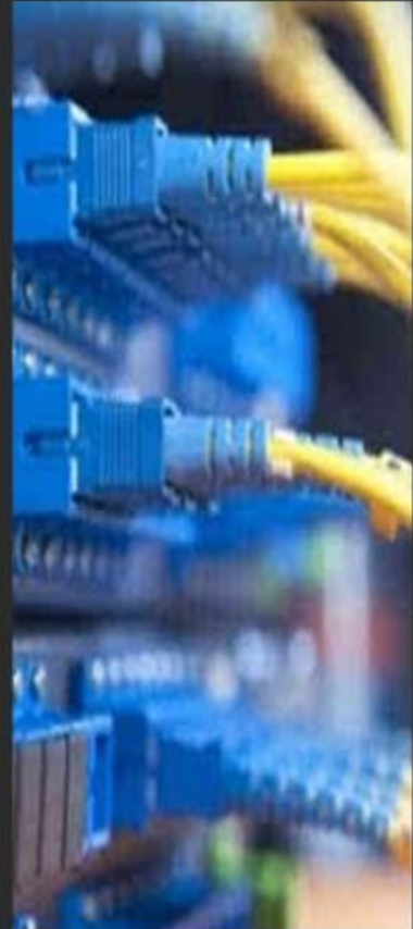
Data Center signal
