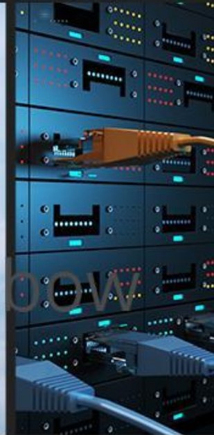
▲ Data Center signal
