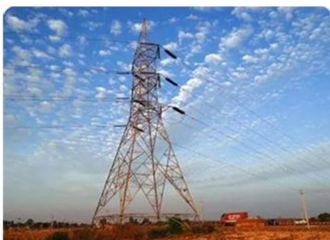
Field power cable
